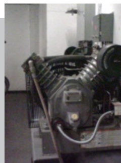
Air Compressor – Full Visible
